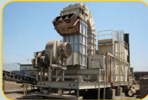
Our LTTD facility is conveniently located in Azusa, California near the 605 and 210 freeways.
