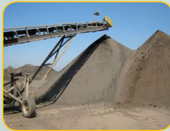
Our Azusa, CA facility can receive up to 2,500 tons of soil per day.
